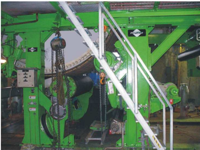
Photo 1 PM#5 press section after modernization
